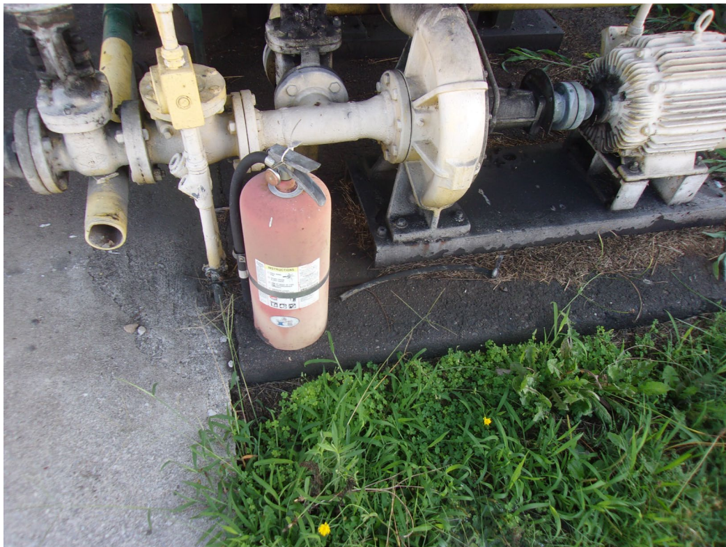
Photo #10: View of the stained pavement.
